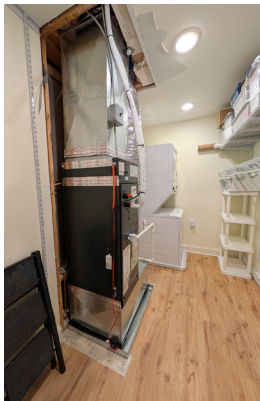
New heat pump looms large in a closet Photo by Alexandra Doumani.
